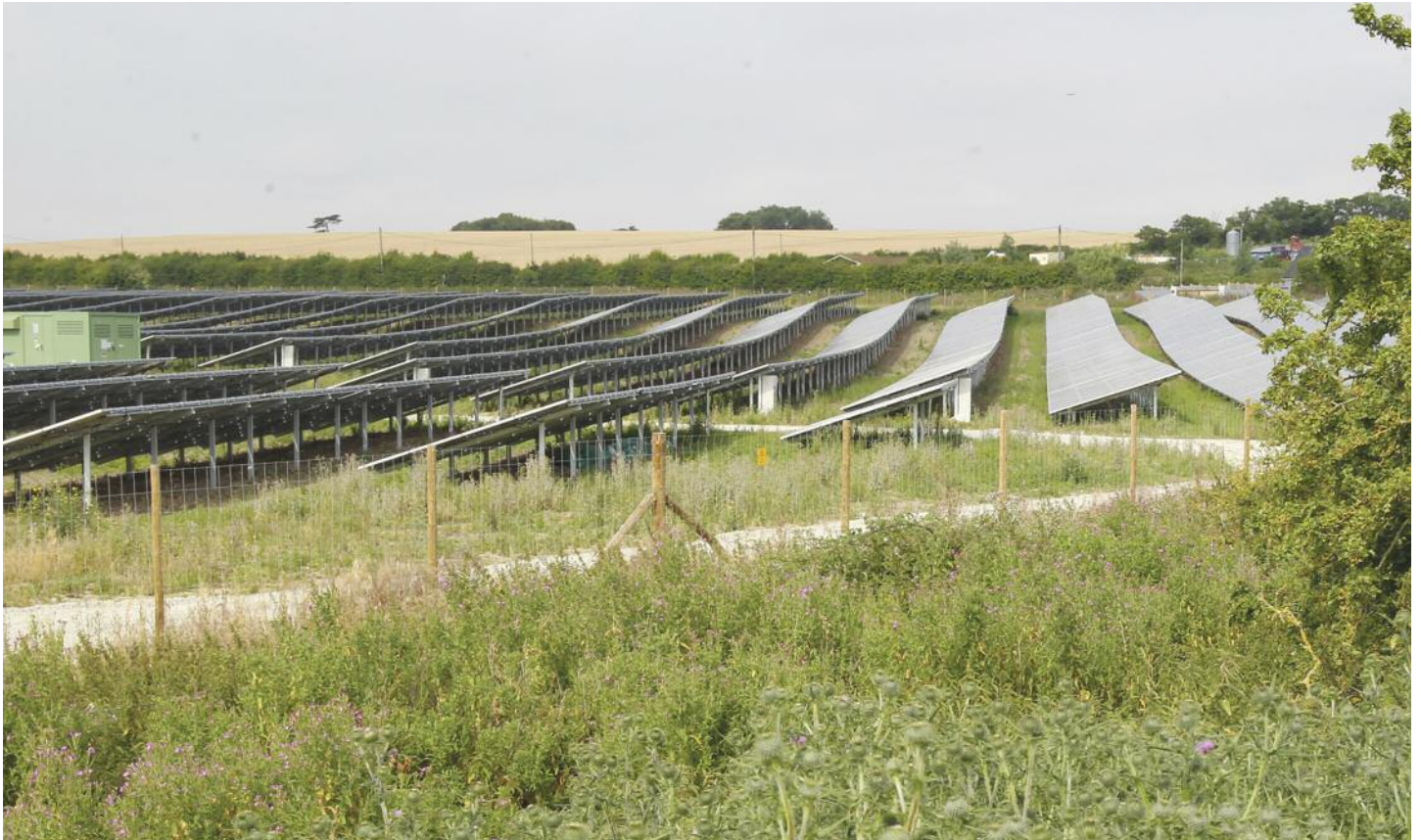
Orchard Farm Solar Array
